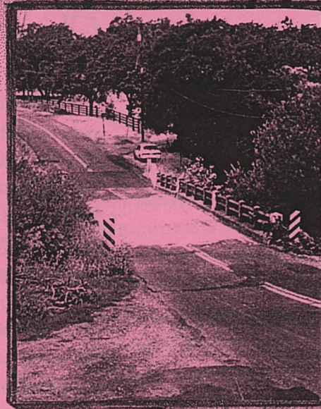
A view of the Grange Road Bridge. Construction is now scheduled to begin sometime in 1999.
